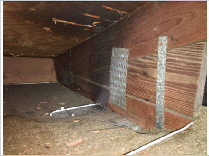
Toe Nail - Not Meeting Nail Requirements
